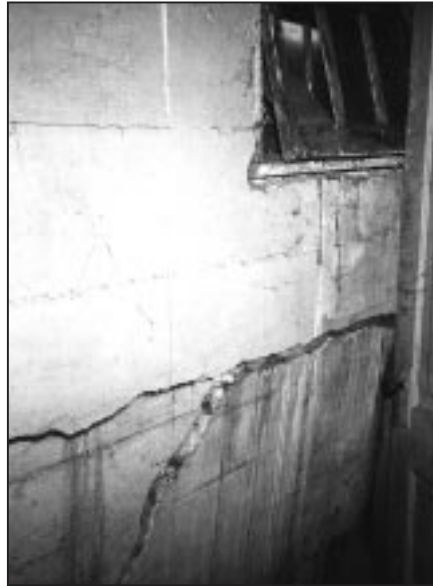
Figure 2-8 The walls of this basement in North Dakota failed because of the pressure exerted by water and saturated soil.
